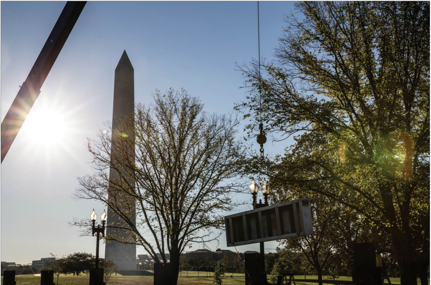
INSTALLING A CLOSURE SYSTEM FOR A LEVEE SYSTEM NEAR THE NATIONAL MALL IN WASHINGTON, D.C. (SOURCE: USACE/ALFREDO BARRAZA, HTTPS://FLIC.KR/P/NCOSTC ).
