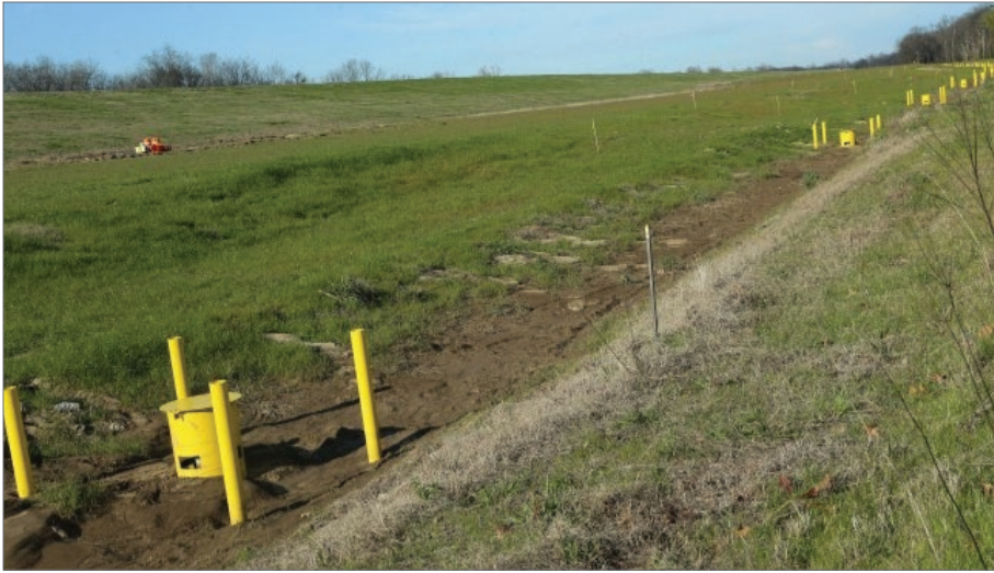
RELIEF WELLS ALONG THE MISSISSIPPI RIVER INSTALLED SINCE THE 2011 FLOOD EVENT (SOURCE: USACE).
