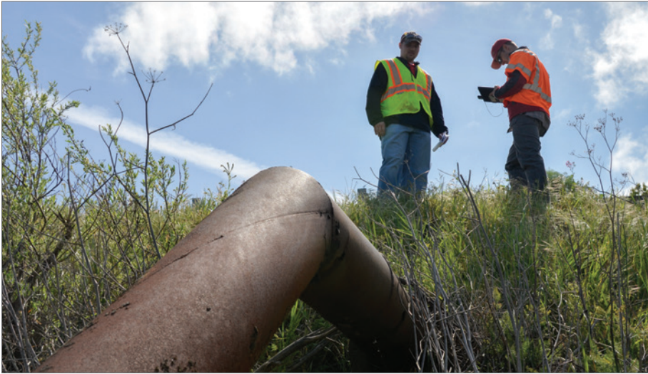
USACE LEVEE INSPECTORS INSPECT THE CONDITION OF A PIPE DURING A ROUTINE LEVEE INSPECTION ON THE SACRAMENTO RIVER, CALIFORNIA (SOURCE: USACE/CHRIS GRAY-GARCIA, HTTPS://FLIC.KR/P/E6LDQ6 ).
