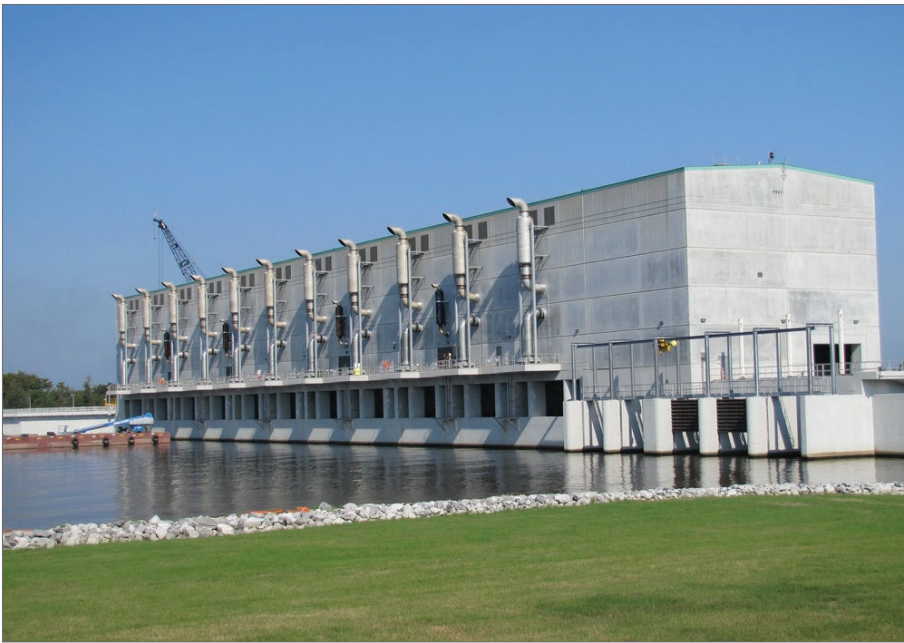
THE PUMP STATION AT THE WEST CLOSURE COMPLEX IN NEW ORLEANS, LA; THIS IS THE LARGEST DRAINAGE PUMP STATION IN THE WORLD (SOURCE: USACE).
