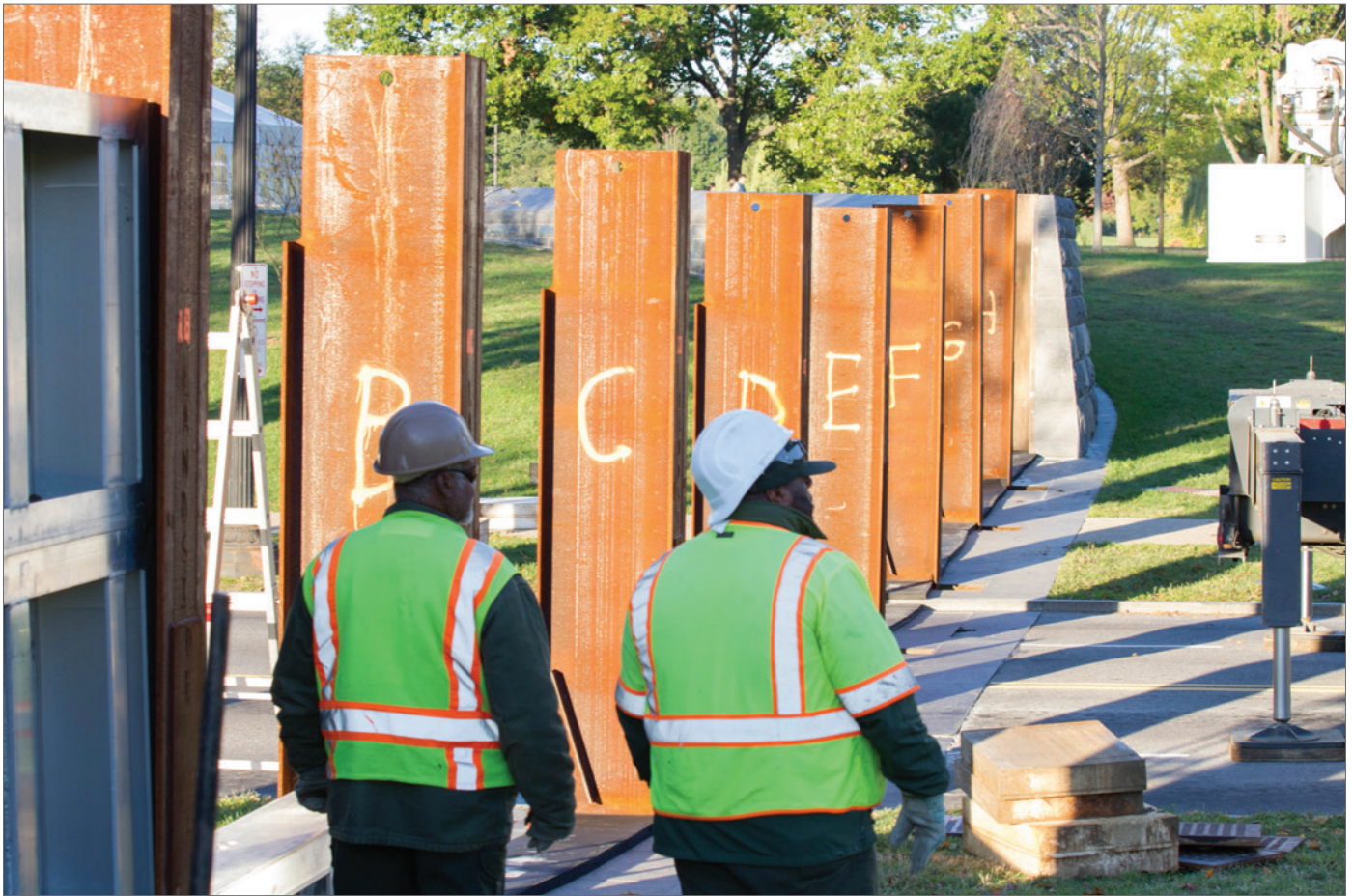
ANNUAL TESTING OF THE WASHINGTON, D.C., 17TH ST CLOSURE ENSURES THE STRUCTURE CAN BE ERECTED PROPERLY IN THE EVENT OF HIGH WATER (SOURCE: USACE/ALFREDO BARRAZA, HTTPS://FLIC.KR/P/NCOMZD ).
